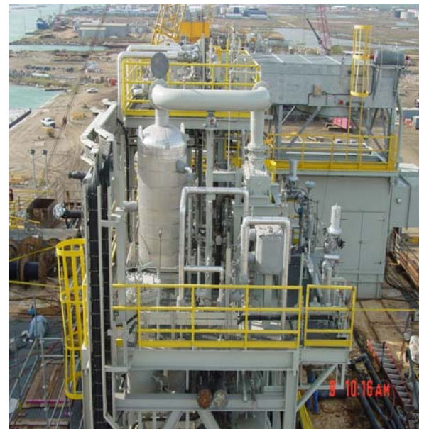
Reclaimer for KMG Red Hawk in the Gulf of Mexico. The first floating cell-spar design
