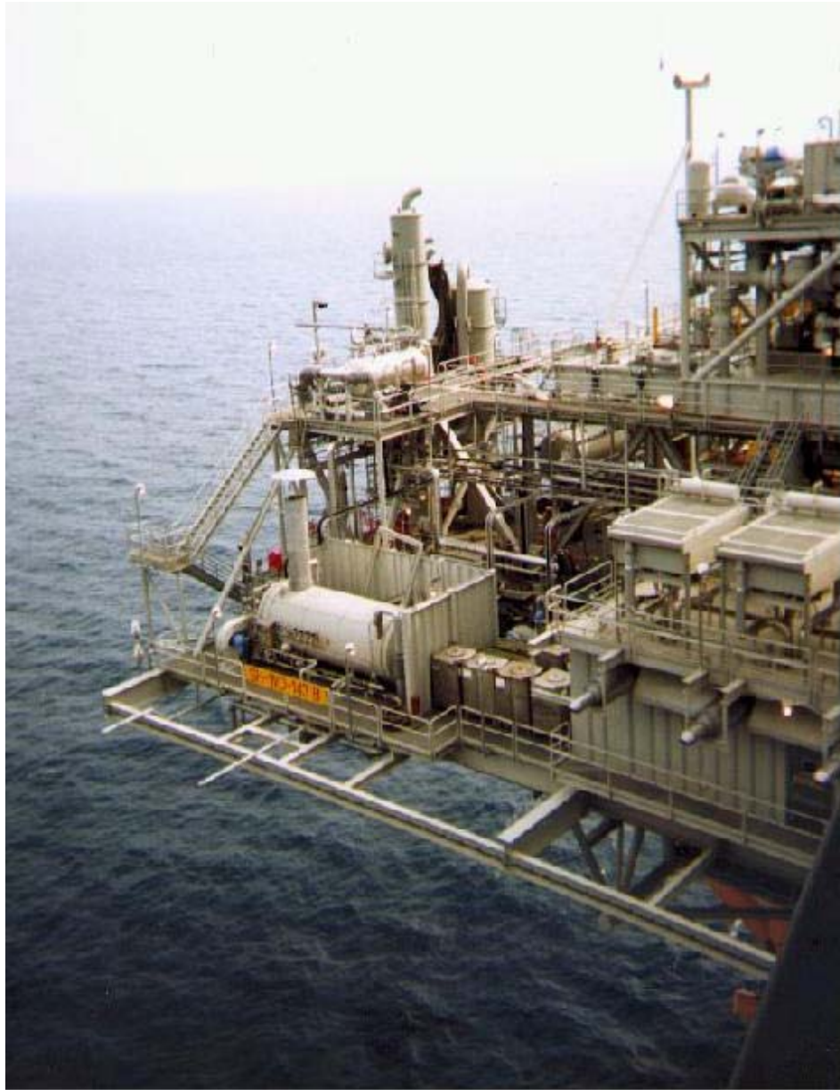
Figure 3 Photograph of Glycol Regeneration/Reclamation Unit
